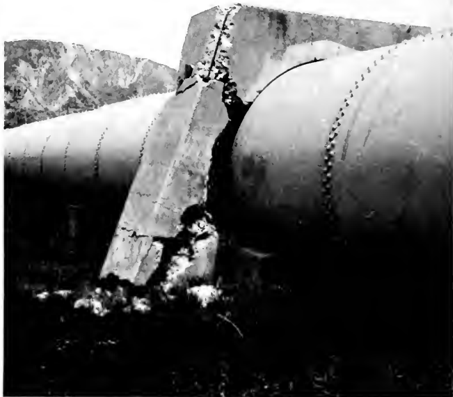
Photo 2. First Los Angeles Aqueduct penstock. Shattered anchorage pier just north of Upper Van Norman Reservoir.
